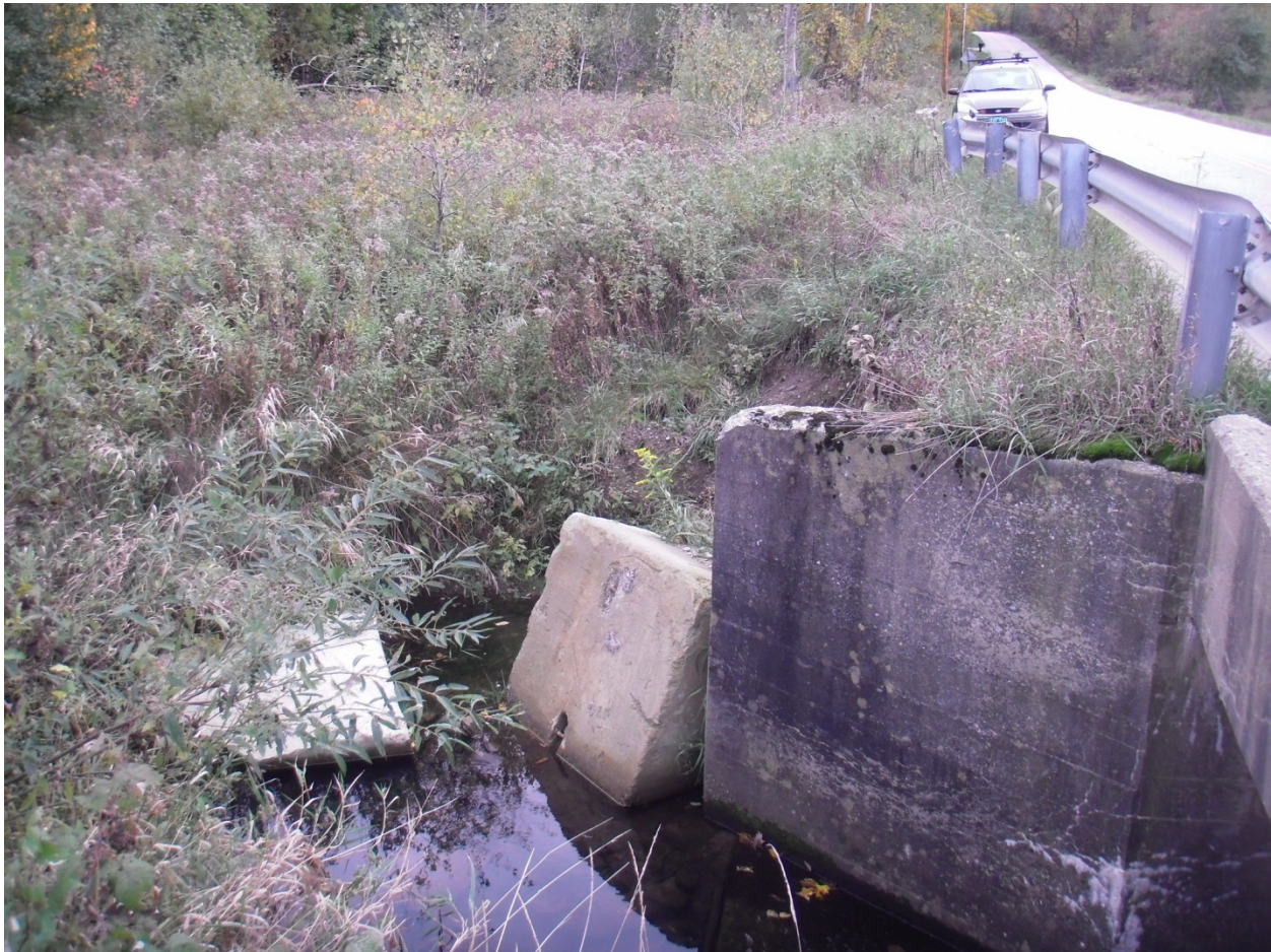
Figure 6. Failing slope near inlet to box culvert over Mill River on Oakland Station Rd.
