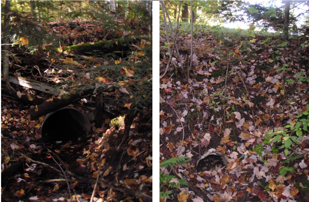
Figure 20. Partially clogged culverts with unstable cover slopes.
