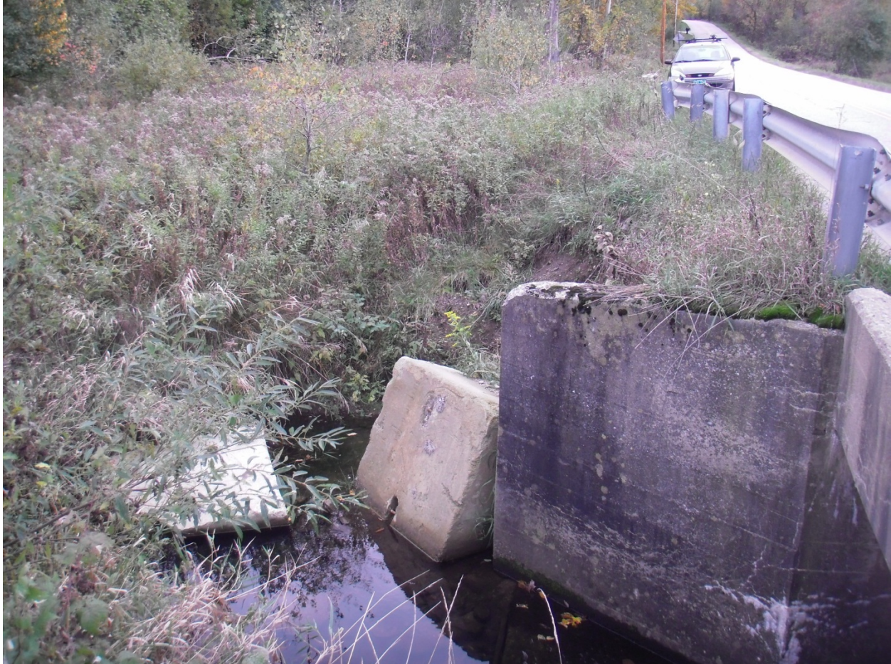
Figure 21. Failing slope near inlet to box culvert over Mill River on Oakland Station Rd.
