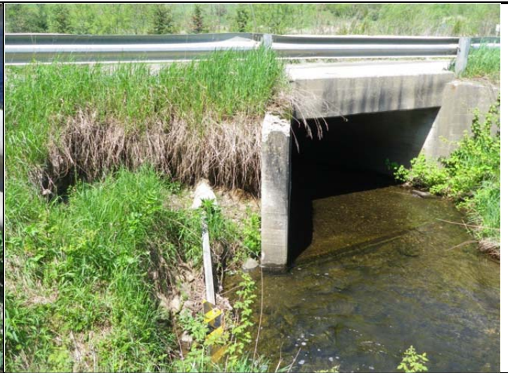
Photo 2. Looking downstream at bank erosion
