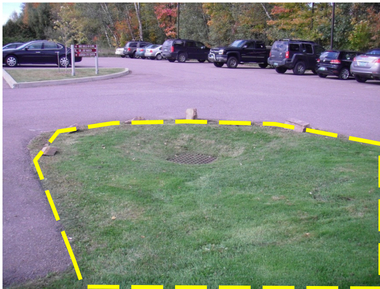
Figure 4. Existing catch basin that could be retrofitted and integrated into a stormwater treatment practice.
