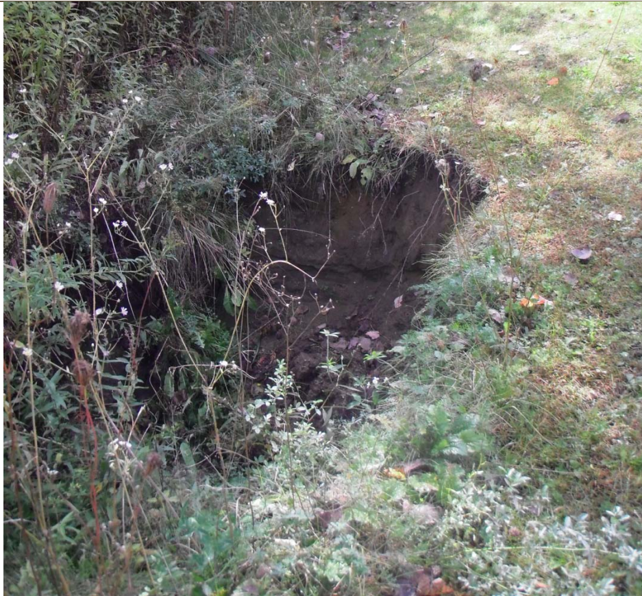
Figure 16. Headcut in road side ditch at the bottom of Lakeview Terrace.
