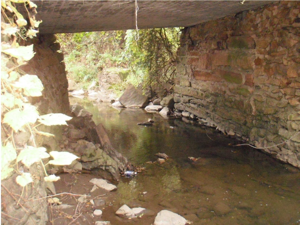
Figure 7. Deteriorating stone abutments of Mill River Rd. bridge over Rugg Brook.
