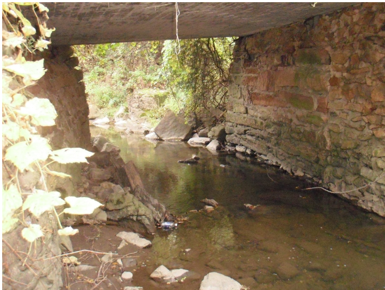
Figure 22. Deteriorating stone abutments of Mill River Rd. bridge over Rugg Brook.
